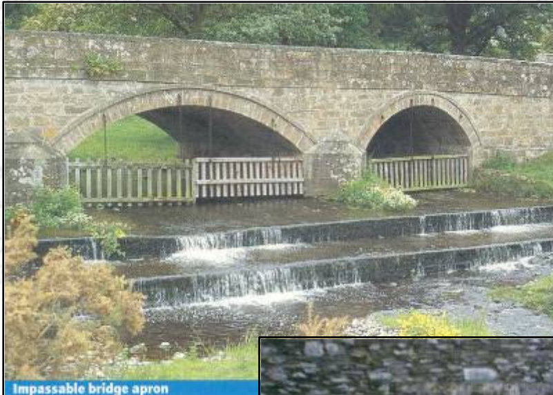
Impassable bridge apron
